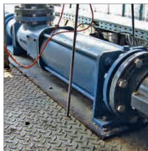
Pumping substrate between fermenters
