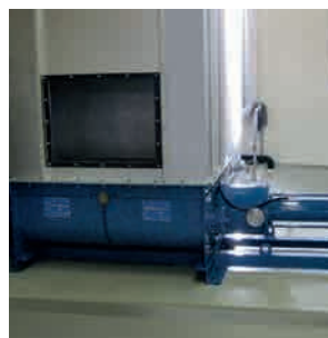
Conveyance of dewatered sewage sludge from decanter for drying: KL65R80.2 Triplex progressing cavity pump
